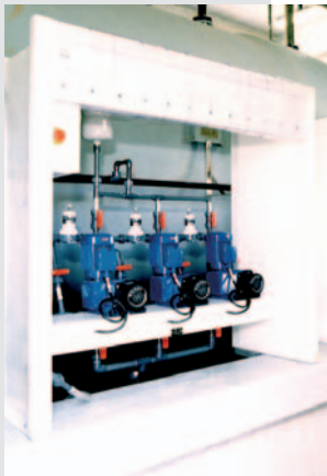
Dosing pumps integrated in a dosing skid for water treatment
